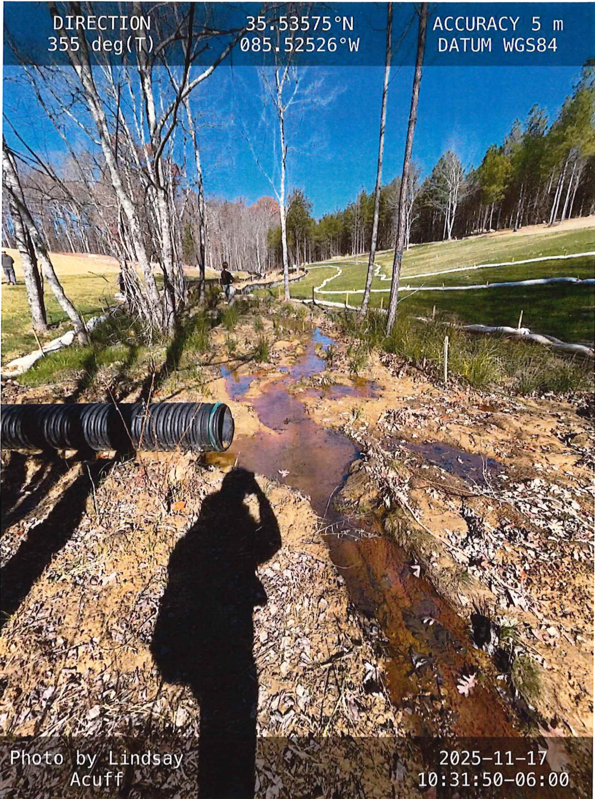
Photo 5: Unauthorized pipe discharging construction stormwater into stream channel outside of permit area.
