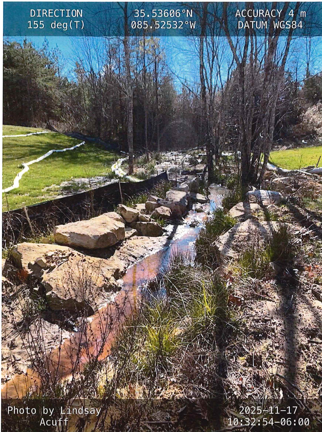
Photo 4: Stream channel altered with sedimentation and unauthorized rock armoring outside of permit area.
