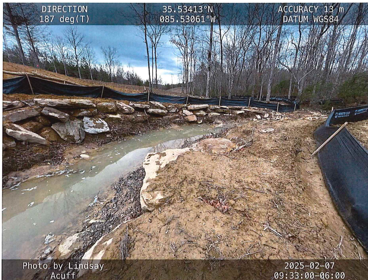
Photo 1: Unpermitted alterations to unnamed tributary of Little He Creek.
