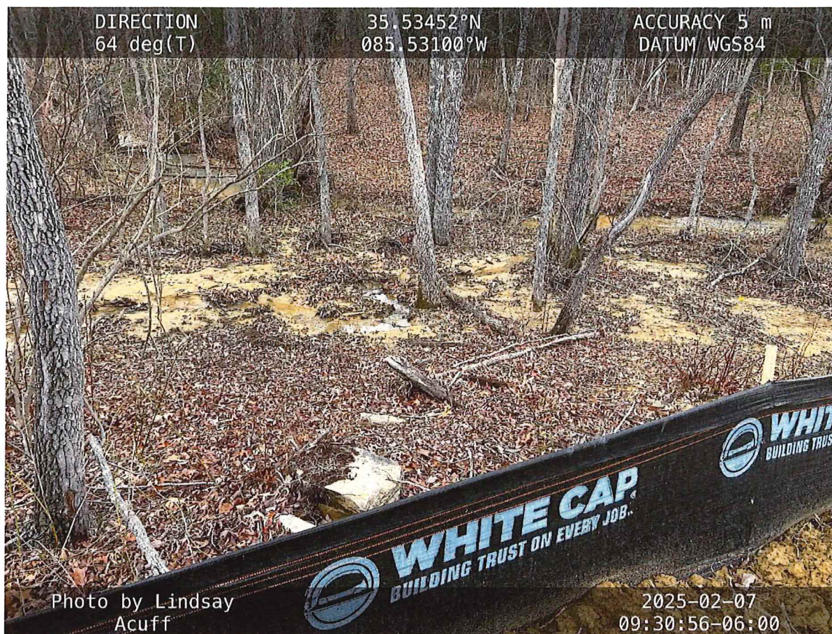
Photo 4: Silt fence installed incorrectly, allowing sediment to enter waters of the state.
