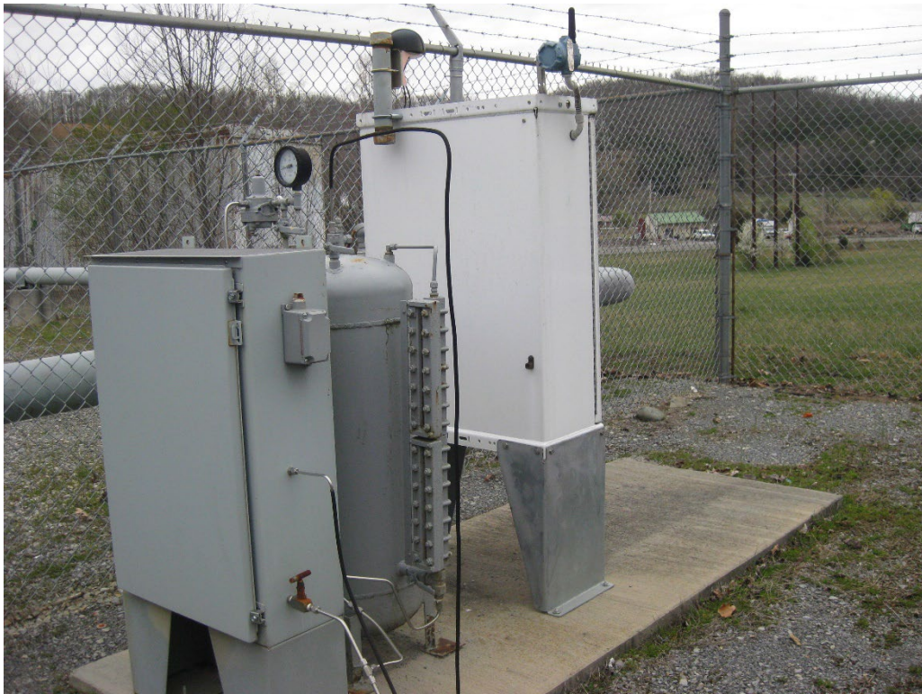
Account 378.00, Measuring and Regulating Station Equipment Deodorant Tank
