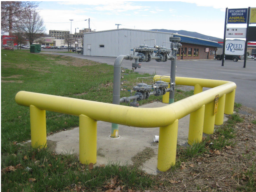
Account 378.00, Measuring and Regulating Station Equipment Overview
