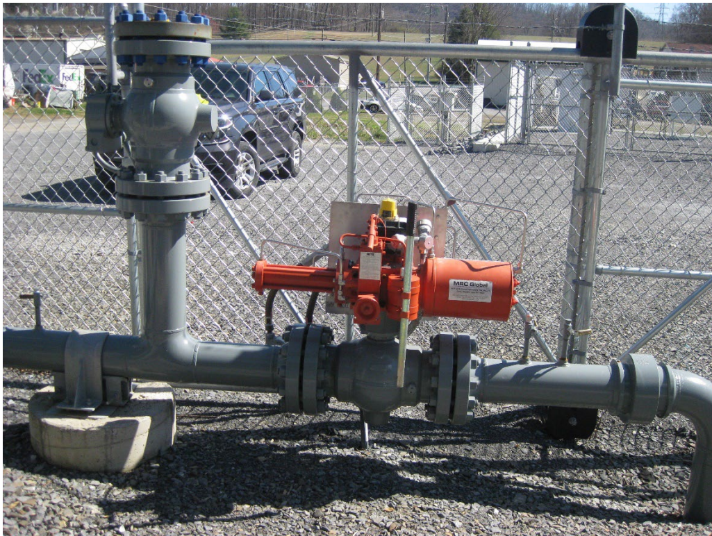
Account 378.00, Measuring and Regulating Station Equipment Remote Operated Valve (ROV)
