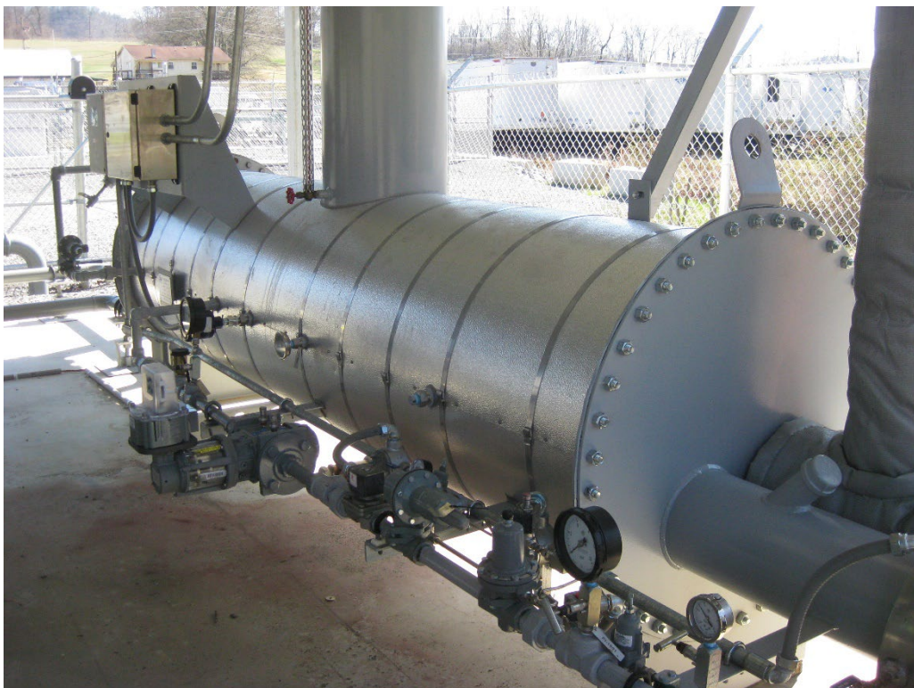
Account 378.00, Measuring and Regulating Station Equipment Heater
