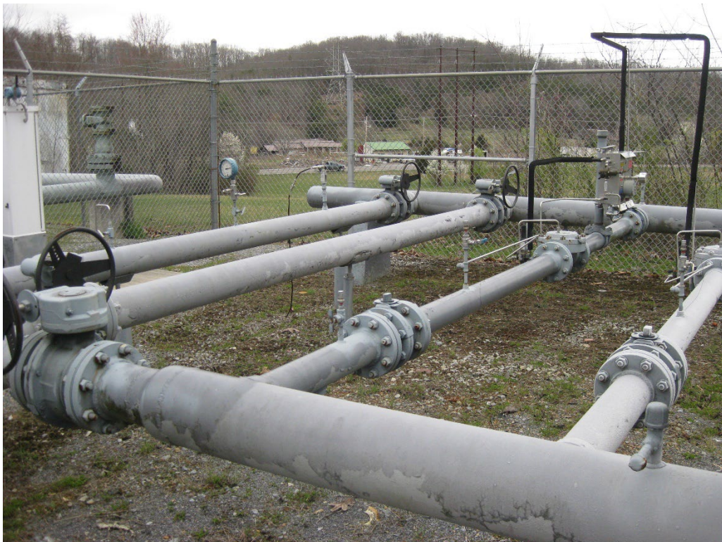
Account 378.00, Measuring and Regulating Station Equipment Regulator Runs
