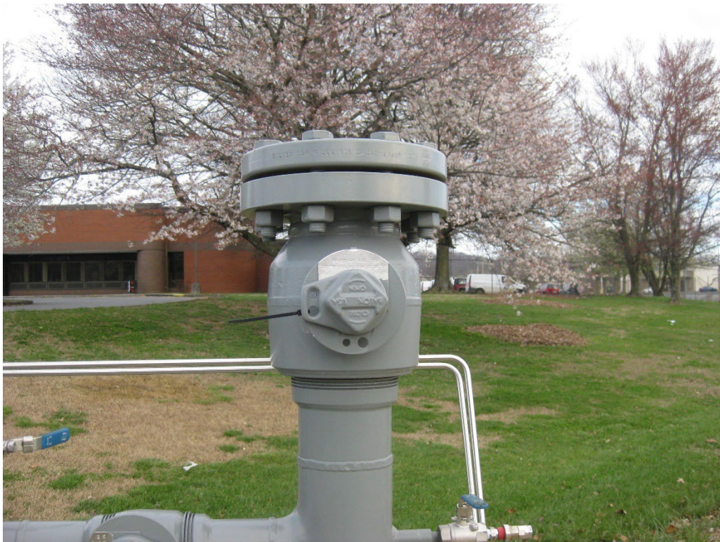
Account 378.00, Measuring and Regulating Station Equipment Relief Valve
