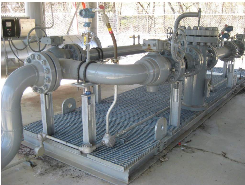
Account 378.00, Measuring and Regulating Station Equipment Metering (Left Unit)
