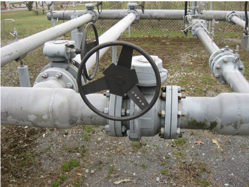
Account 378.00, Measuring and Regulating Station Equipment Valves
