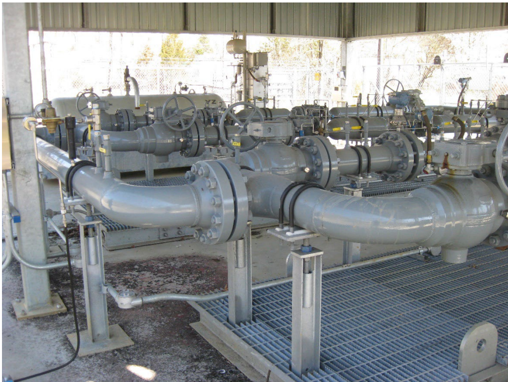
Account 378.00, Measuring and Regulating Station Equipment Two Regulator Runs
