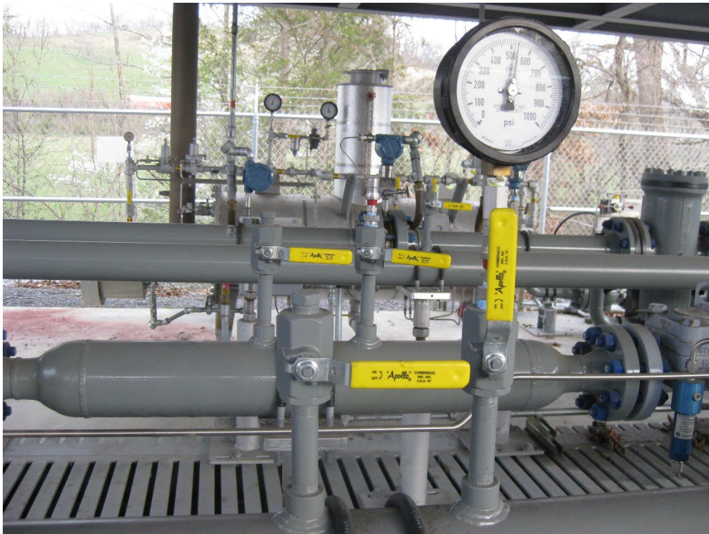
Account 379.00, Measuring and Regulating Station Equipment - City Gate Valves
