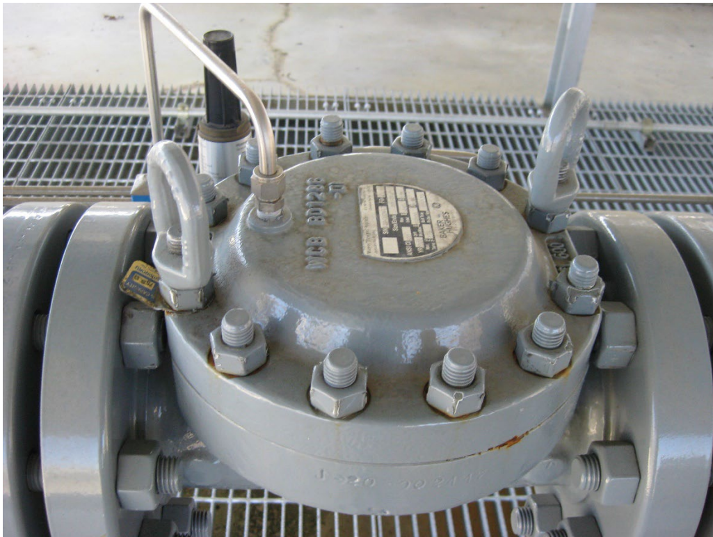
Account 378.00, Measuring and Regulating Station Equipment Mooney Flowgrid Regulator
