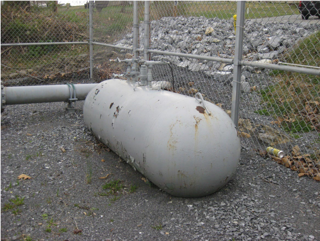
Account 378.00, Measuring and Regulating Station Equipment Decommissioned Storage Tank
