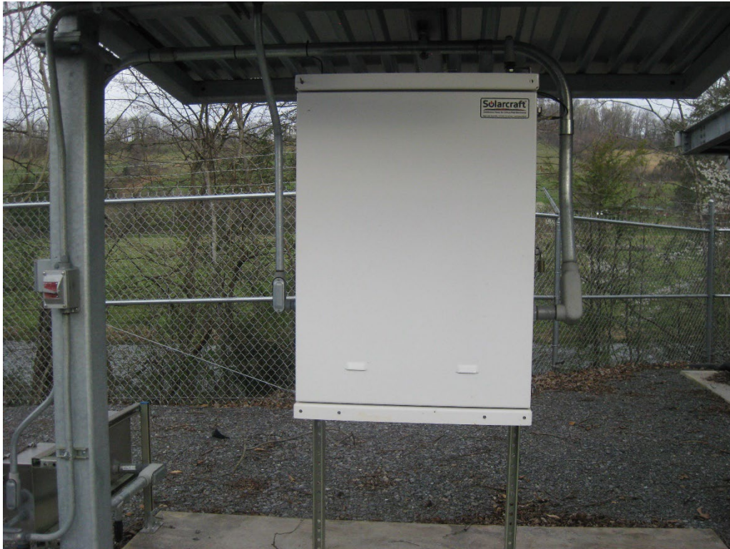
Account 379.00, Measuring and Regulating Station Equipment - City Gate Information/Communications
