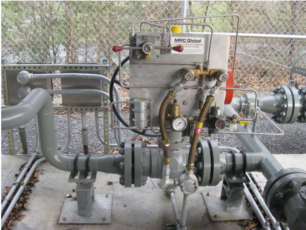
Account 379.00, Measuring and Regulating Station Equipment - City Gate Remote Operated Valve (ROV)
