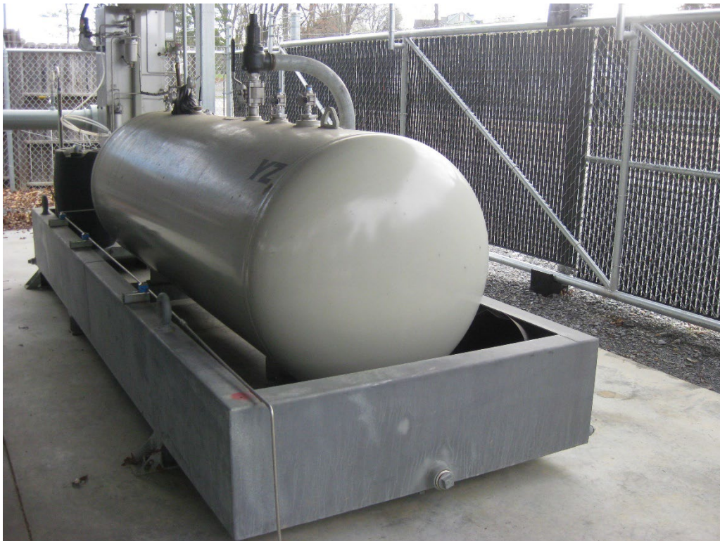
Account 379.00, Measuring and Regulating Station Equipment - City Gate Deodorant Tank
