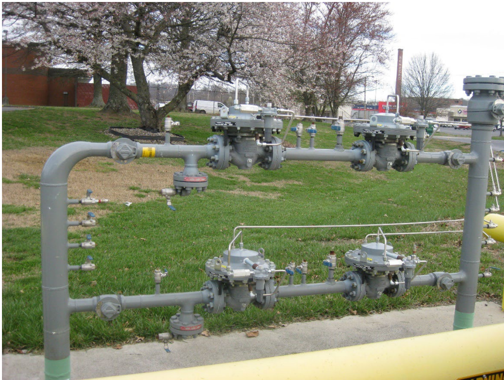
Account 378.00, Measuring and Regulating Station Equipment Regulator Run
