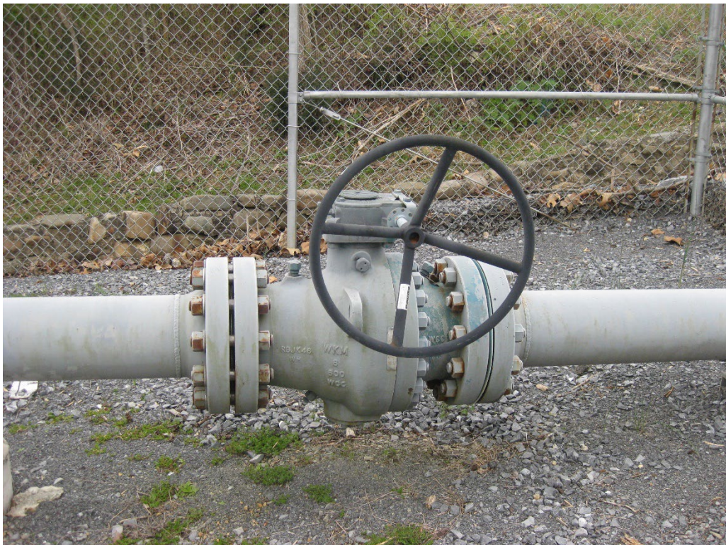
Account 378.00, Measuring and Regulating Station Equipment Distribution System
