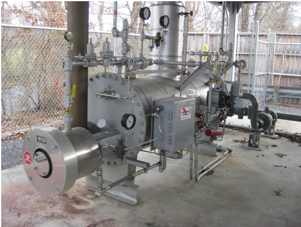
Account 379.00, Measuring and Regulating Station Equipment - City Gate Heater
