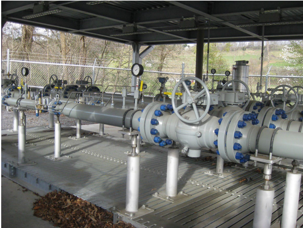
Account 379.00, Measuring and Regulating Station Equipment - City Gate Regulator Runs
