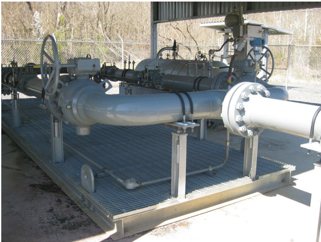
Account 378.00, Measuring and Regulating Station Equipment Regulator (Right Unit)
