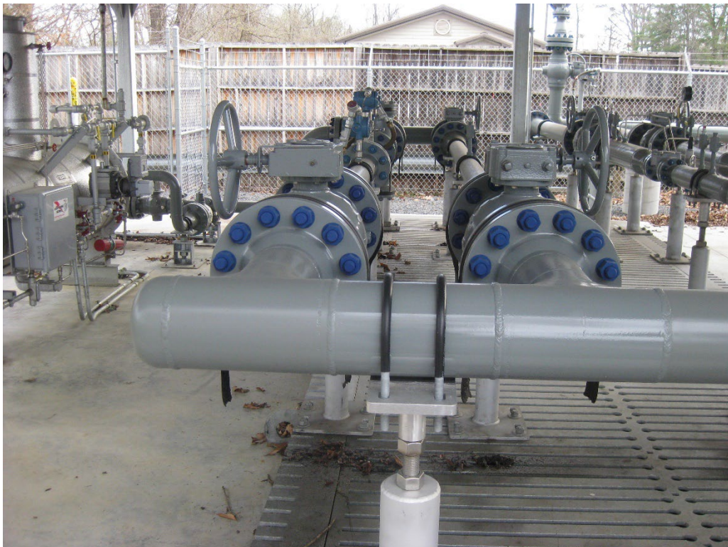
Account 379.00, Measuring and Regulating Station Equipment - City Gate Regulator Run
