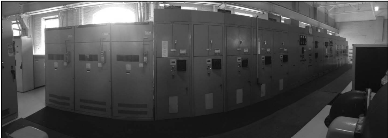
Exhibit 5-6 Medium Voltage Switchgear
