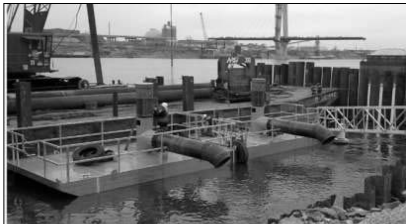
Figure 1 Example Floating Pump Station
