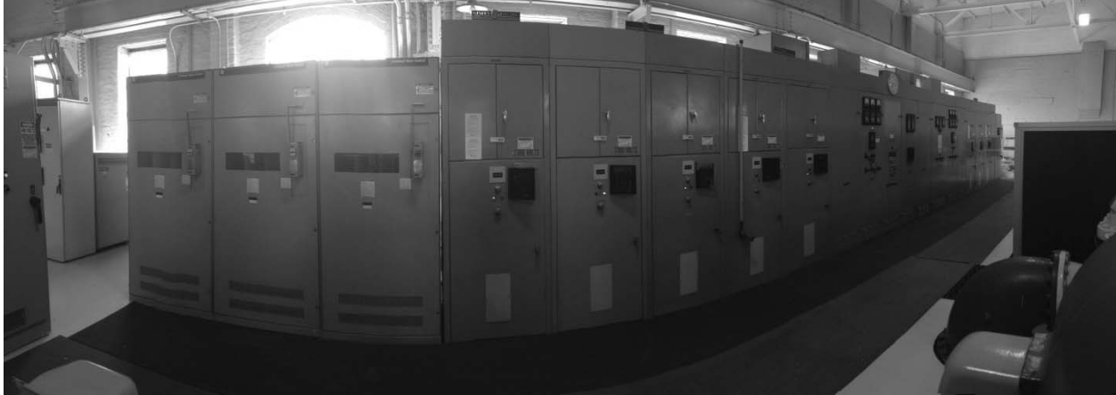
View of Existing Medium Voltage Switchgear Lineup
