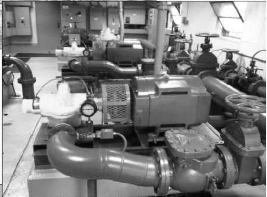
South Mission Ridge Pumps ▶
