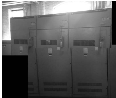
Individually served Fusible Switches units associated with power and motor controller feeds
